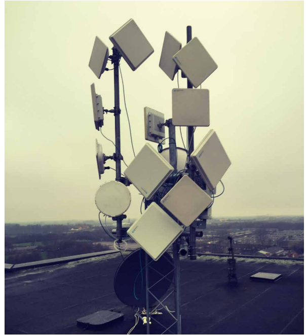
Figure 4 - SyncMaster and Trinity PtP and PtMP links in operation.
